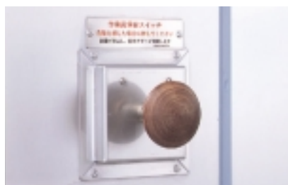
Operator safety switch
